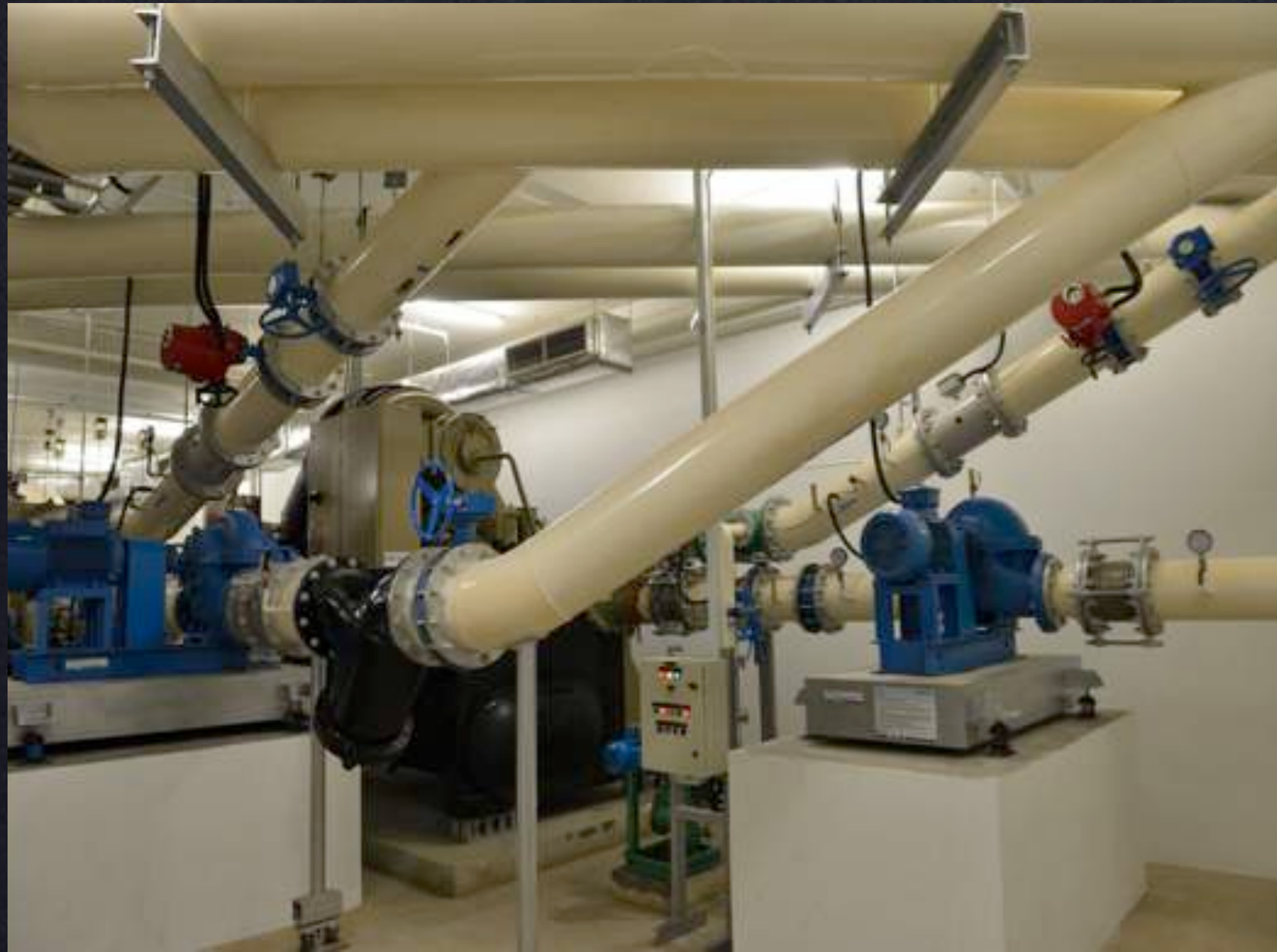
Big pipes, small pumps
